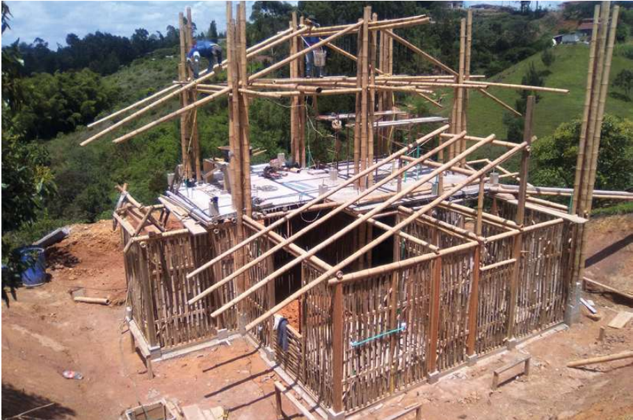
fig.76 the whole building, in the phase of the construction of the second floor and roof structure.
