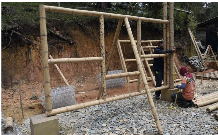
fig.82 the guadua-frame of a wall is being constructed. The main columns are built on concrete bases.
