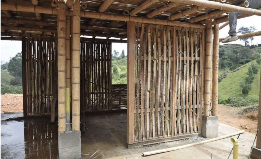
fig.75 the ground floor of the construction with the main column structure made of guadua on a concrete base. In the picture, we can see the walls made out of a wooden frame and guadua pieces.
