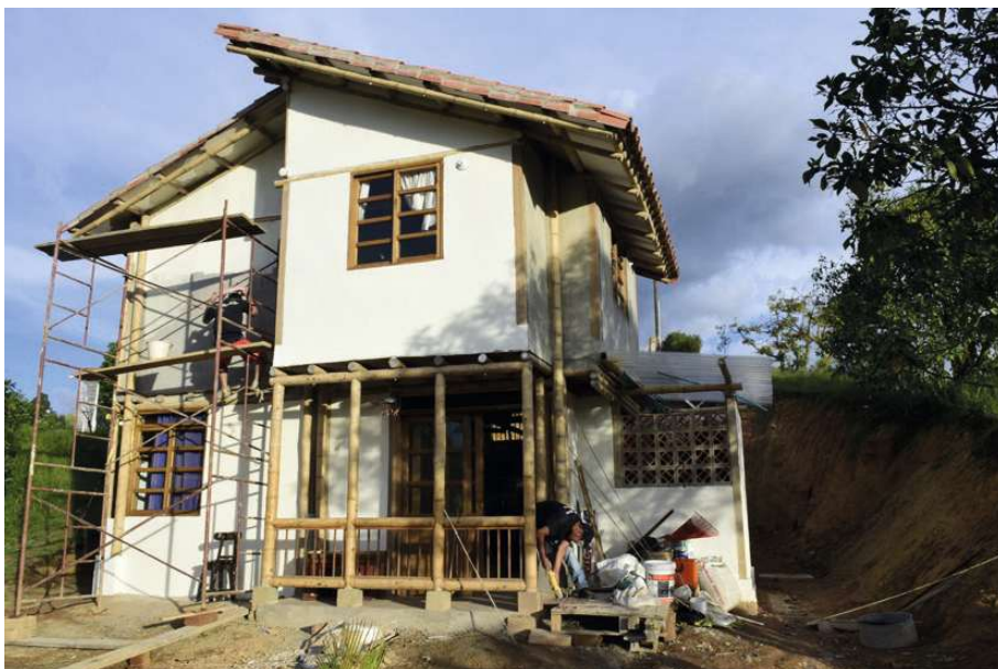
fig.78 the whole building, in the last phase of the construction, with already painted walls.
