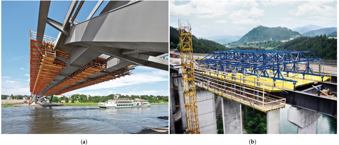
Figure 1. Construction techniques for deck slabs with CIP concrete. Photos courtesy of Peri SE, Germany (a) and Doka GmbH, Austria (b). (a) Stationary formwork attached to the steel structure. (b) Formwork carriage on a roller support system.
