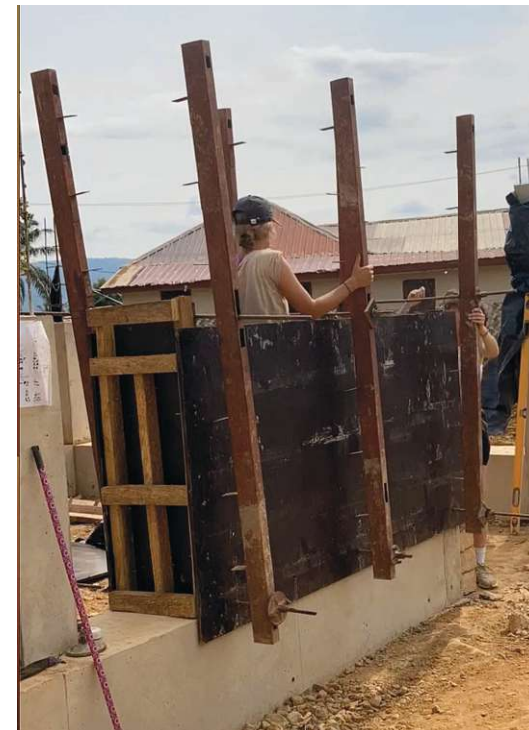
Fig.189: Sideboards and Headboards were screwed together, and vertical metal upstands were added
