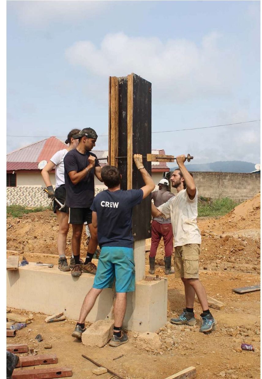
Fig.147: Setting up the formwork for the second part of the reinforced concrete columns | Week 5
