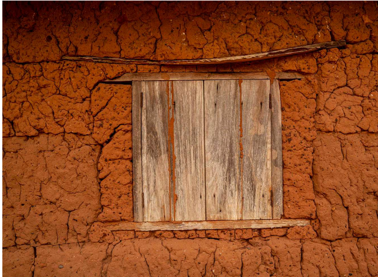
Fig.59: Window detail | Wood is used as a lintel during and after construction | Eastern Region
