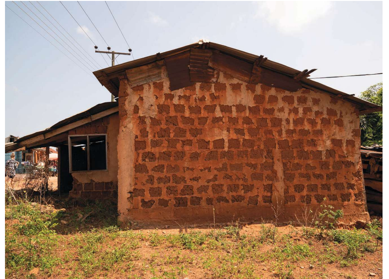
Fig.63: Atakpamé wall, which at first sight looks like an earth brick wall because of the plaster in Eastern Region
