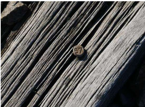
Date nail from 1957 on deteriorated wooden sleeper.
