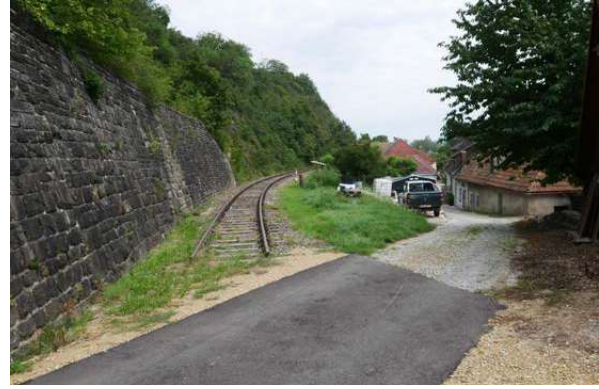
KM 38.7 End of intact trackage a
