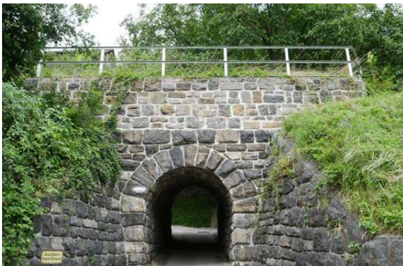
KM 38.8: Stone arch underpass, structure is in good condition and recently renovated
