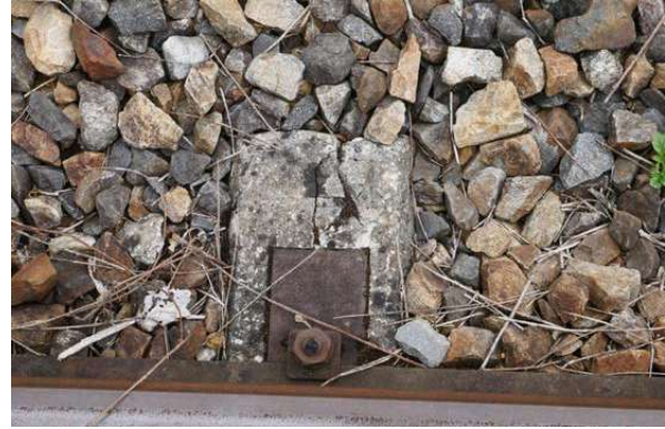
Condition of sleepers in this section vary, some two block concrete sleepers exist and area in poor condition.
