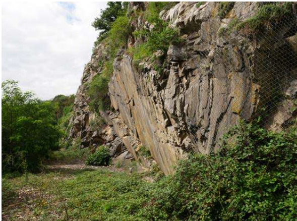
KM 49.5: Unstable rock faces with partial metal netting.
