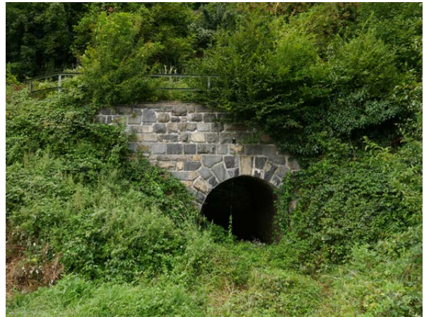
KM 51.1: Second small stone arch bridge, appears in good but unrenovated condition.
