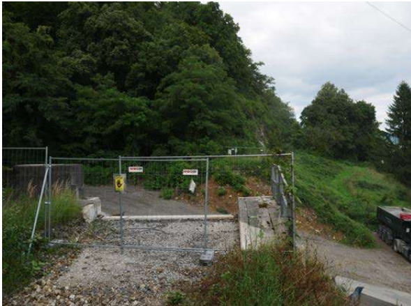
KM 52.4: Concrete bridge at entry to quarry demolished for better truck access
