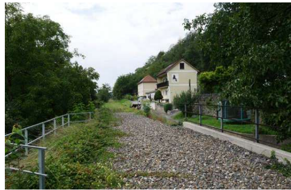
KM 38.8: Right of way and track level details of stone arch underpass
