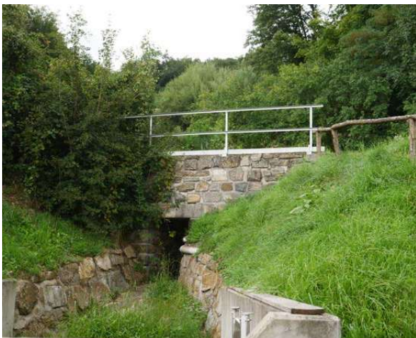
KM 49.9: Small stone box culvert. Culvert appears in good condition and recently renovated
