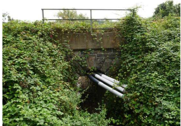
KM 50.9: Small arch culvert. Structure appears to be in good shape but heavily overgrown
