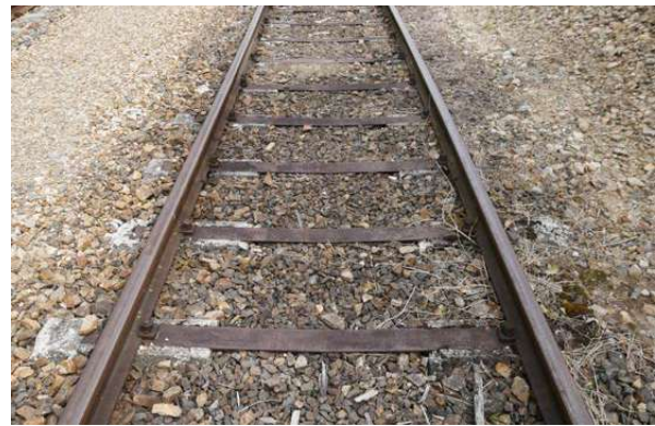
Example of the twin block concrete sleepers that were problematic for continued operation of the middle segment
