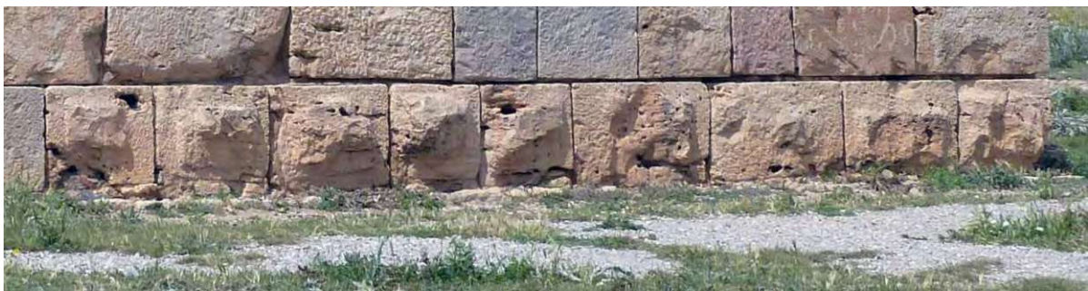
Figure 13 Red marked area zoomed in, displaying various states of drafted margins, in Masinissas Tomb, Algeria
