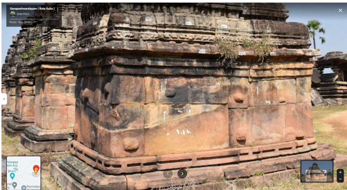
Figure 56 Another perspective of the same structure in Ghanpur temples (Kota Gullu), India
