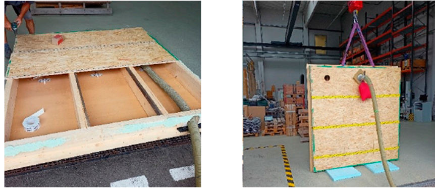
Figure 6. Horizontal position before blowing in (left) and vertical position before blowing in (right).
