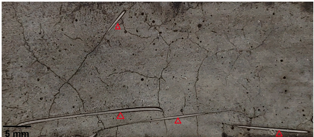
Fig. 7. Example of a cracked surface (Δ: fibers).
