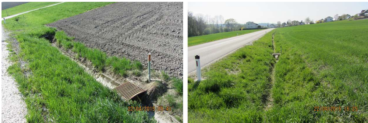
Fig. 3.3: Roadside ditch with multiple storm drains at varying distances. The left picture was taken upstream of the right.
