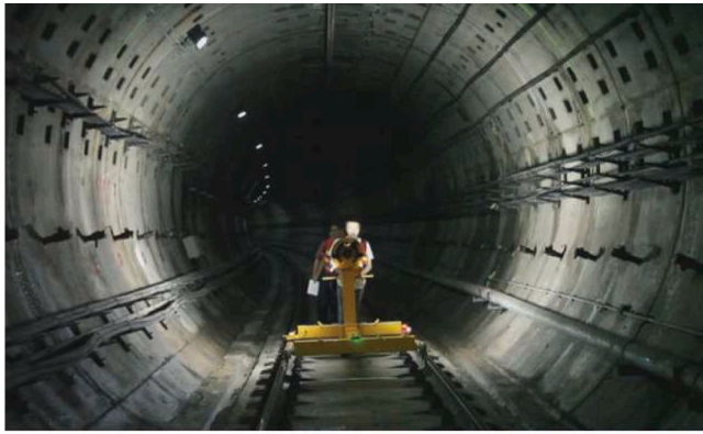
Fig. 10. Segmental tunnel lining of Metro Line 7 in Shanghai, consisting of tubbing rings with aligned longitudinal joints; a rail-bound vehicle, equipped with non-metric CCD cameras, was used for inspection of the tunnel by Ai and Yuan (2019).
