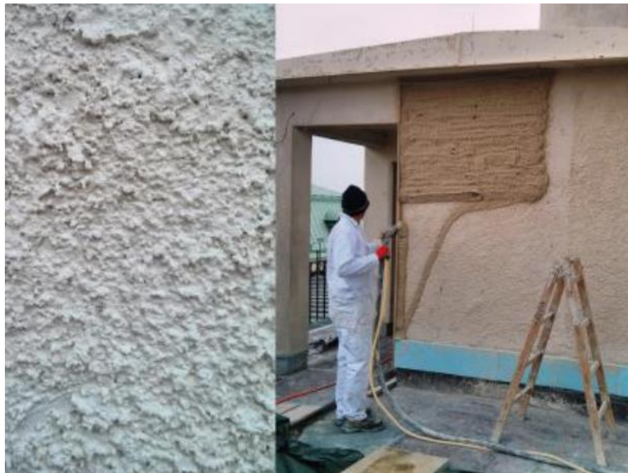
Figure 11: Adhesive primer (on the left), application of FIXIT 222 with a plastering machine (on the right) (Proskurnina, n.d.)
