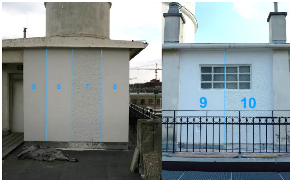
Figure 8: View of the test areas on the south façade (fields 1-4), west façade (fields 5-8), and north façade (fields 9-10) (Schuss et al. 2017)
