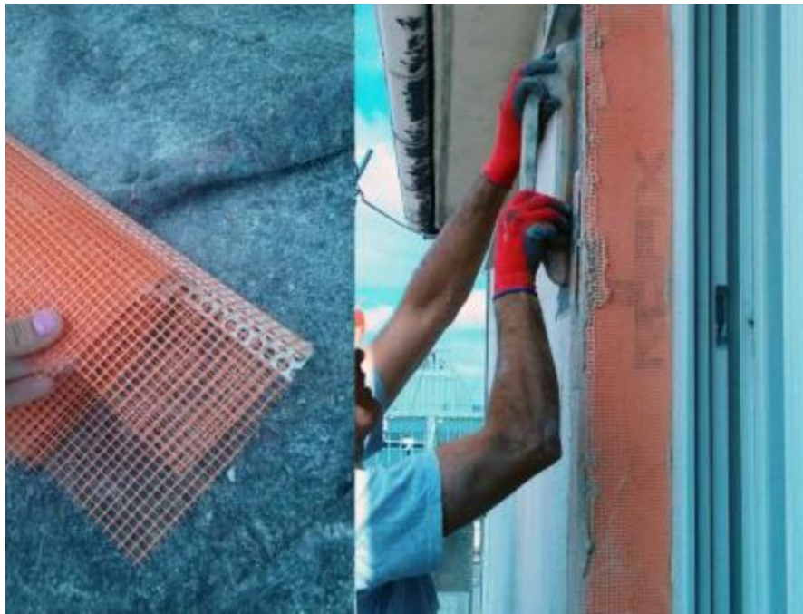
Figure 13: Reinforcement mesh for corners of opening (left), application of reinforcement mesh (right) (Proskurnina, n.d.)
