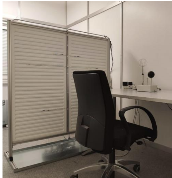
Figure 39: Test room equipped with a cooling panel
