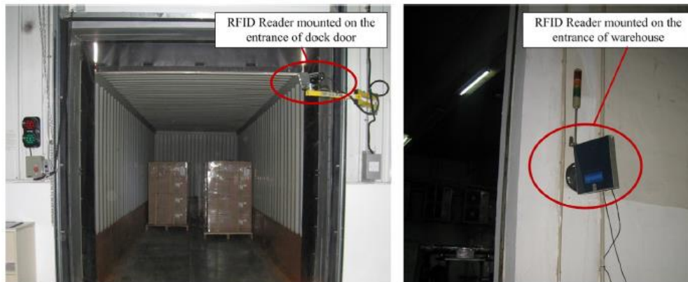
Figure 85: Passive RFID reader mounted on dock door and warehouse entrance
