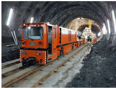
(a) Tunnellokomotive (Quelle: Schöma [85])
