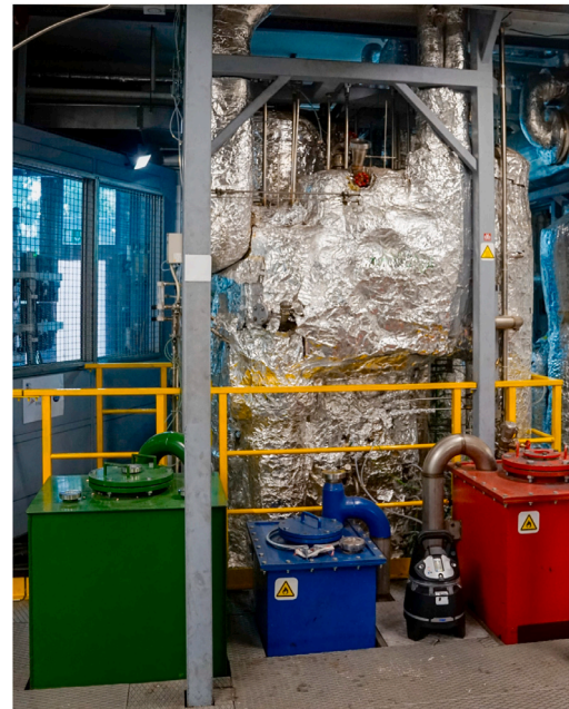
Fig. 2. Upper part of the advanced 100 kW pilot plant at TU Wien.
