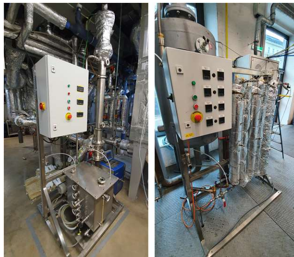
Fig. 4.3: Pictures of the gas cleaning units: RME-scrubber (left) and AC beds (right), reproduced from [38]
