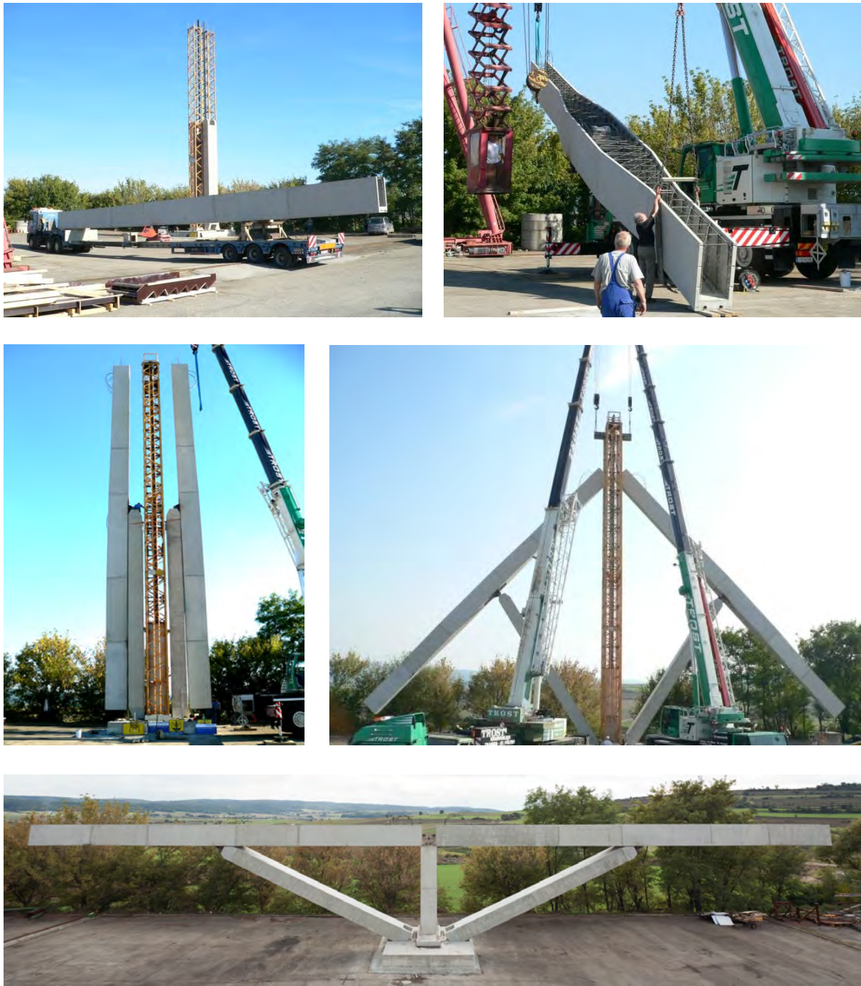
Fig. 2.5: Large-scale testing of the balanced lift method with the application of lightweight thin-walled precast concrete girders (Wimmer (2016))
