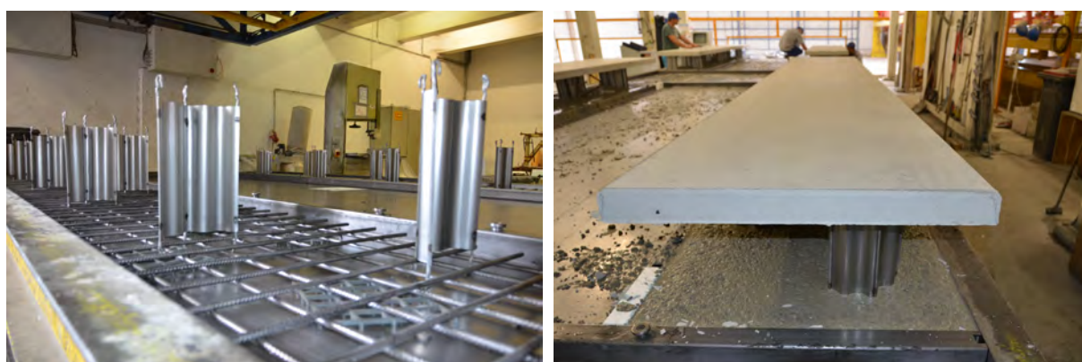
Fig. 4.7: Mesh reinforcement and KAP-steel-waves in place on the formwork for the first panel of the double wall element and the merger of the hardened first double wall panel with the fresh concrete of the second panel.
