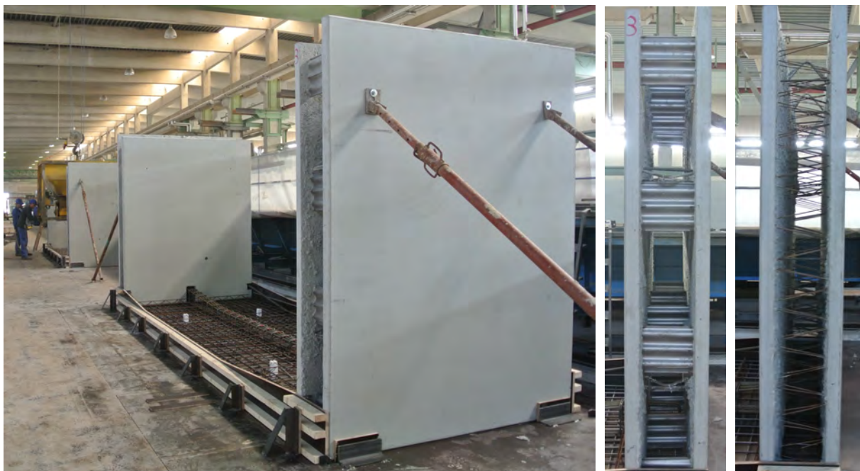
Fig. 6.3: Vertically placed webs of the box-girder section with installed reinforcement cage for the bottom slab. The difference between the reinforcement cages of KAP-steel-wave webs and lattice-girder webs.
