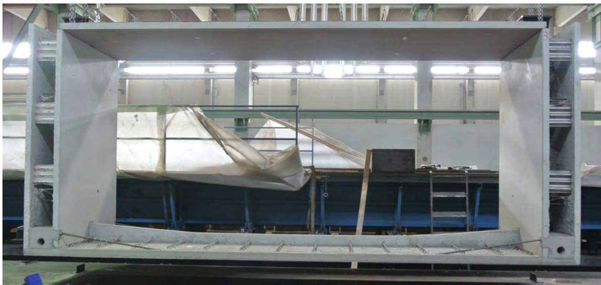
Fig. 6.8: Finished box-sectioned bridge girder out of double wall elements and thin-walled precast elements
