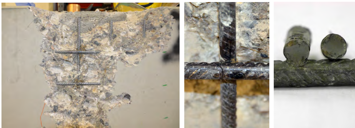
Fig. 4.14: Mesh reinforcement inspection after finished fatigue tests 3 (TS3). Fatigue fracture in mesh reinforcement at tack weld.
