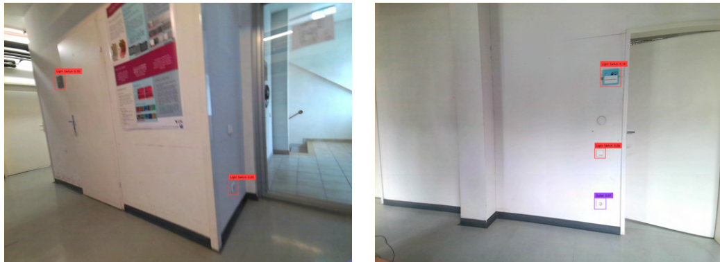
(a) False negative of a light switch. A false positive saves a power socket to be filtered as well. (b) Fire dampers (white circle in the middle) did not respond to any prompt input.
