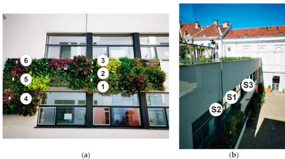
Figure 7. Images of the installed sensors at Schuhmeierplatz School: (a) position of the temperature and humidity sensors in front of the living wall; (b) position of the surface temperature sensors above the living wall, and position of the weather station on the roof terrace.
