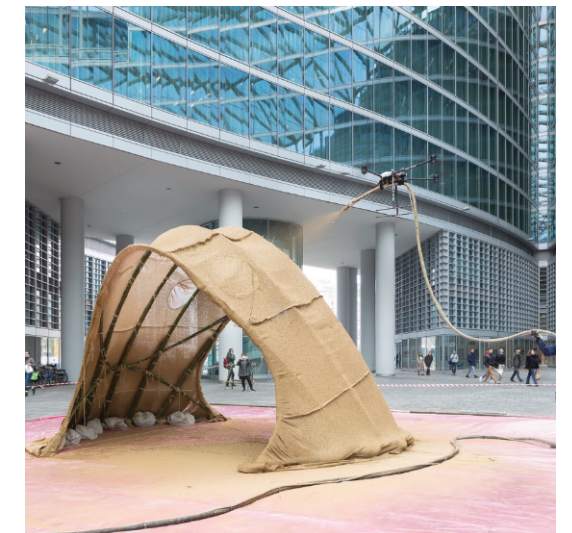
Fig.36. Sands and clays were sprayed on a textile with the help of a drone
