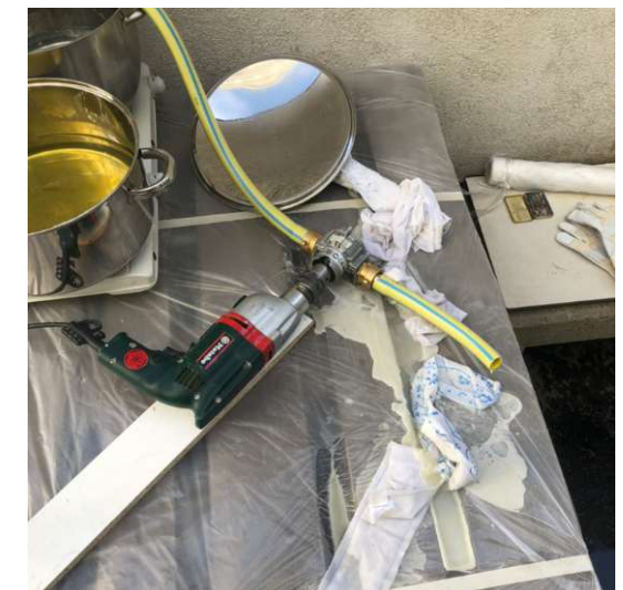
Fig.150. The wax was transferred from the heat source to the formwork with a hose
