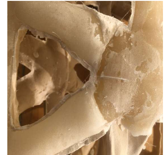
Fig.280. A detail of a casting issue at a joint
