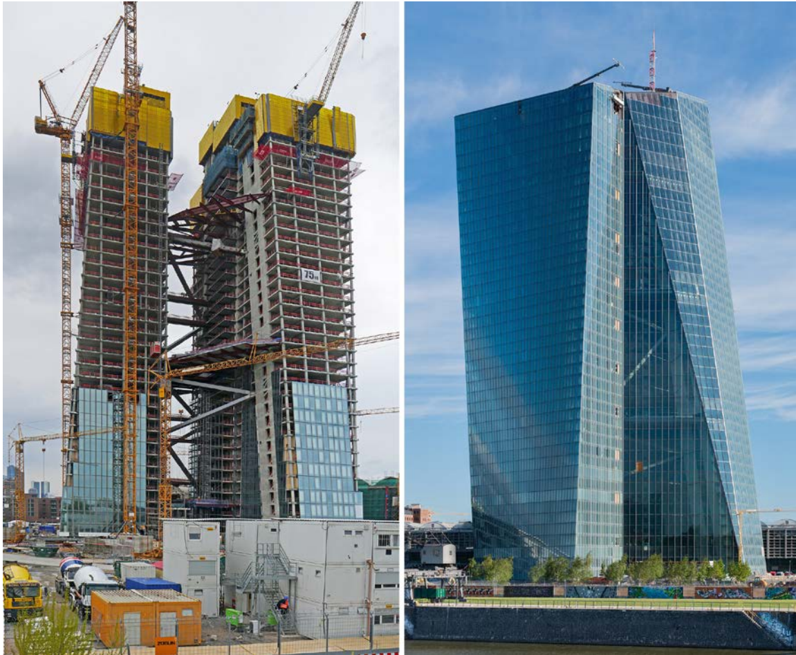
Figure 5. A tall building with an endoskeleton; European Central Bank (ECB), Frankfurt am Main, Germany, 2014, by Coop Himmelb(l)au; left: the endoskeleton is being covered by curtain walls during construction; right: after the construction phase, the endoskeleton is completely covered by curtain walls. Sources/Credits (©): photographs from left to right by Simsalabimbam [50], and Norbert Nagel [51], respectively, via Wikimedia, licensed under CC BY-SA 3.0 (both photographs cropped).
