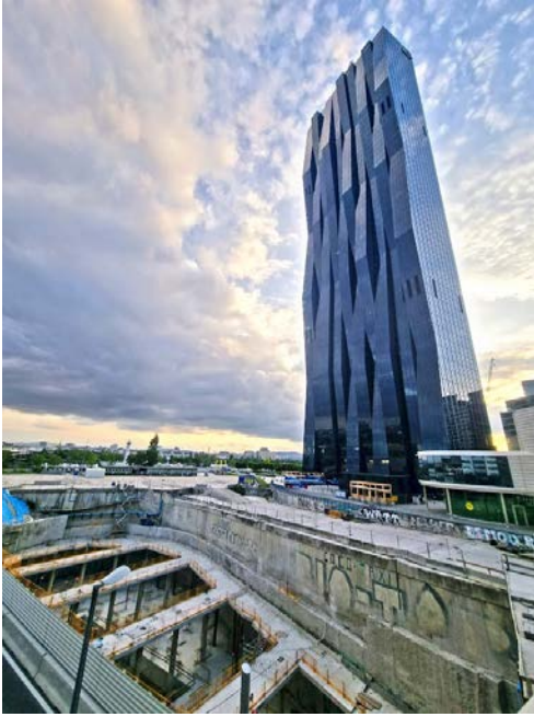
Figure 53. Left: the substructure of DC Tower II in 2023; Right: DC Tower I (completed in 2013) in Vienna, Austria. Source: photograph by the researcher
