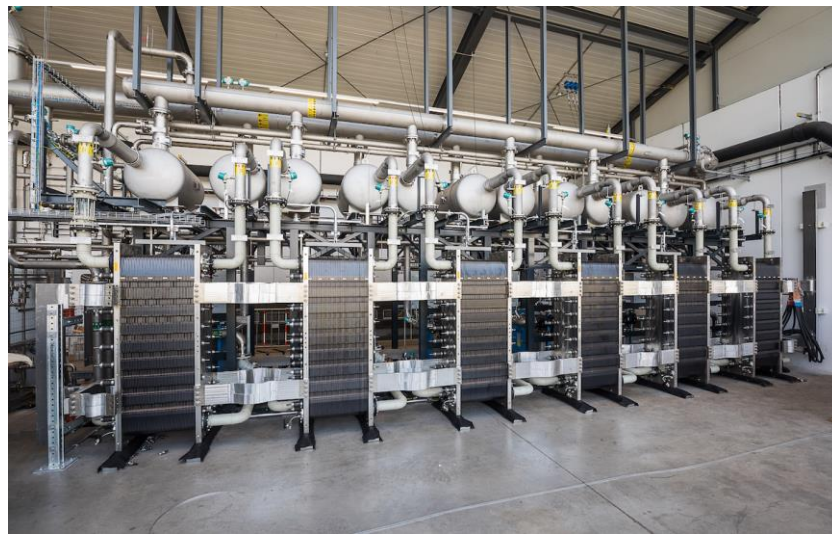
Figure 21: 6 MW array of Siemens Silyzer 300 in Linz, Austria. (Verbund Energy4Business, 2020)
