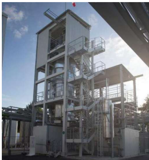
Figure 29: EtoGas Power-to-Gas plant in Werlte, Germany. (Hitachi Zosen INOVA, 2020)
