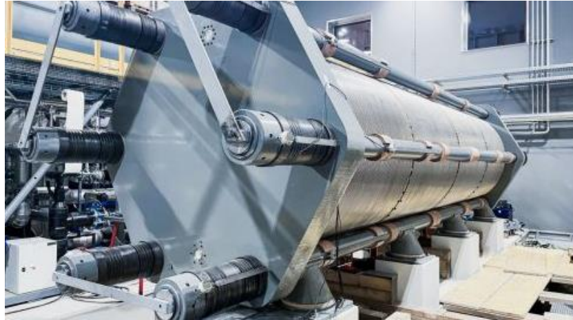
Figure 23: 3.2 MW pressurized alkaline electrolyser Hylink by Sunfire in Völs, Austria. (Demo4Grid, 2022)
