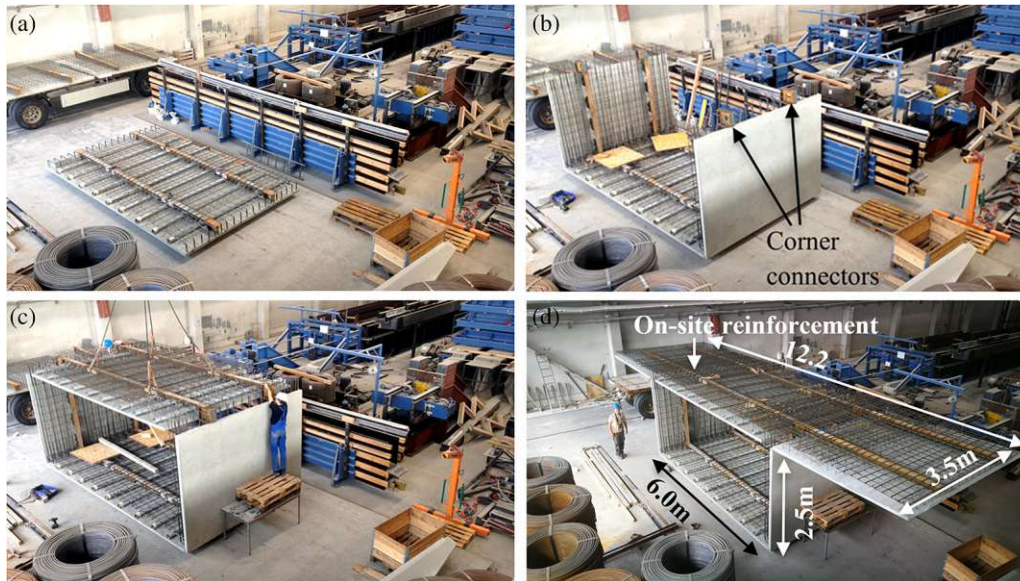
FIGURE 10 Assembly of the segment prototype; (a) placement of the bottom slab in the assembly area; (b) attachment of two web-plates using screw connections on the steel beams; (c) attachment of the deck slab to the top of the web plates; (d) finished segment, including cantilevers
