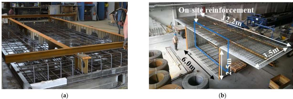
Figure 1. Construction of a lightweight bridge segment using thin-walled prefabricated elements with 70 mm thickness (a) corrugated steel web girders on a casting bed (b) prototype bridge segment with highlighted cross-frame in blue and highlighted surface for shear transmission in orange (taken from [7]).
