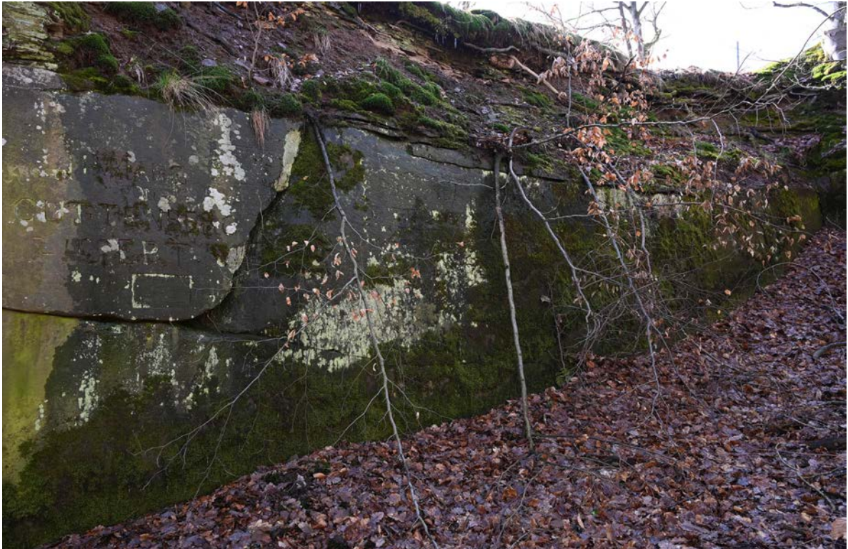
Figure 2. Section of the sandstone wall, highlighting the issues of biological growth.
