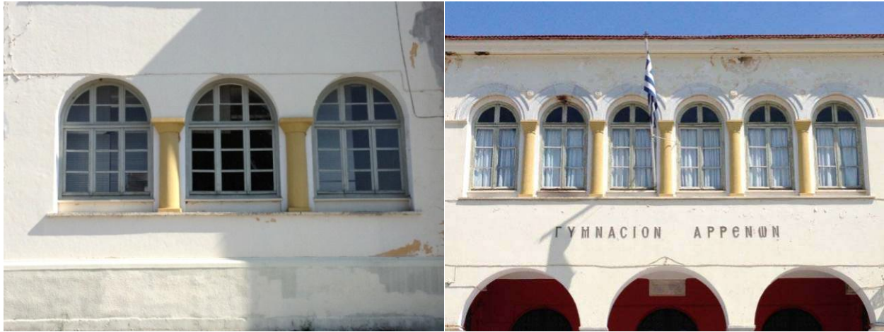
Figures 17,18 Ground floor south facing openings and first floor six windows in a row (Photos by the author, 2019)
