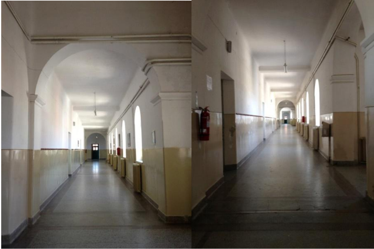
Figures 12,13 Ground floor and first floor north-facing corridors of the west part of the school (Photos by the author, 2019)
