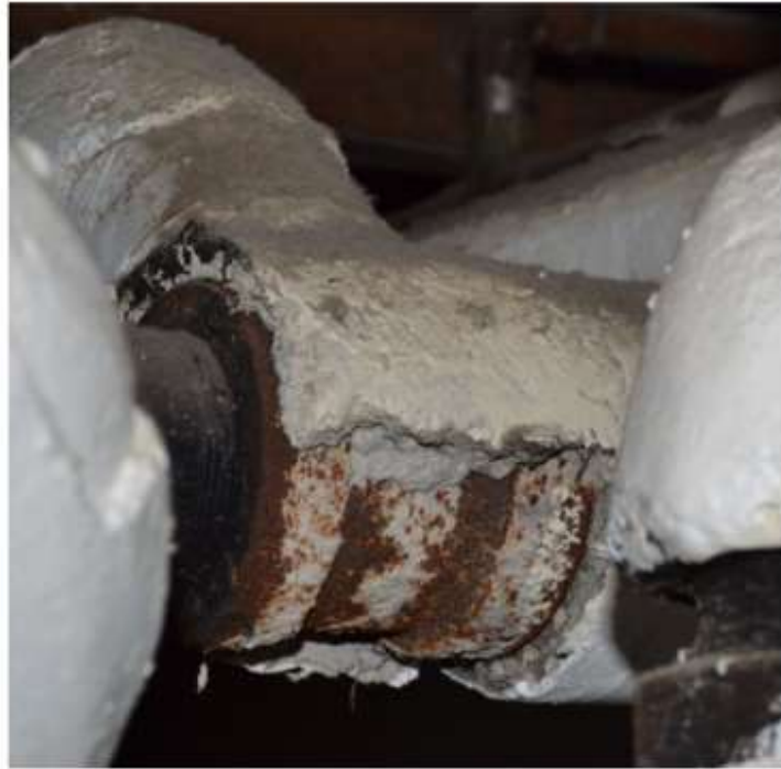
Figure 8 Asbestos pipe wrap (joint partially removed) (source: Asbestos 2021)
