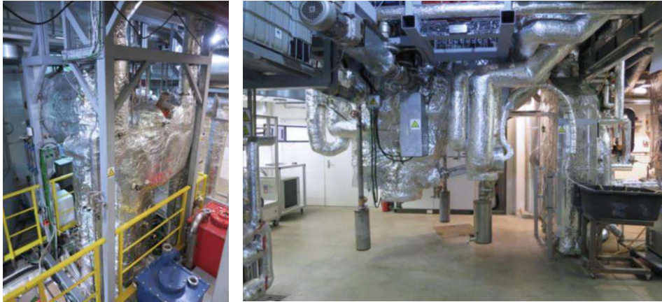
Figure 22: Pictures of the pilot plant including thermal insulation 1
