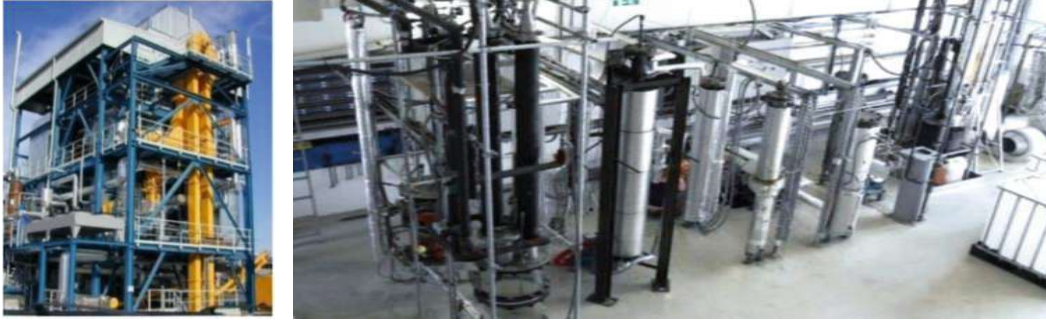
Figure 53: Combined heat and power plant Güssing [TRL9, MRL9] (left); Fischer-Tropsch test plant [TRL 6, MRL 5] 1
