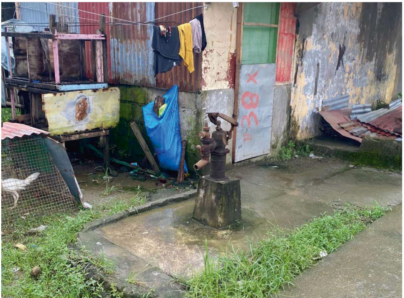
Abbildung 62: Wasserpumpe in Greendale/ Guadalupe
