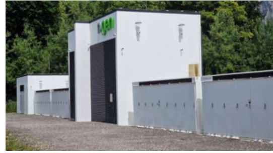
Figure 46 - 20,6 MWh battery storage plant
