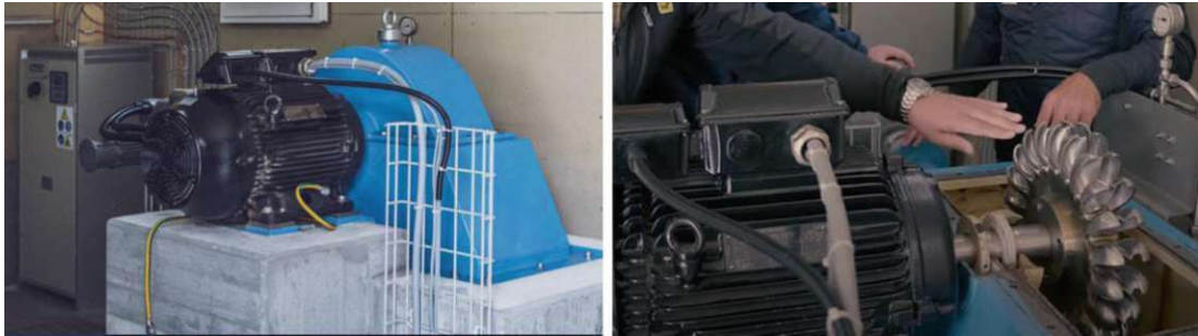
Figure 47 - small turbine/generator of Davos ski resort [13]
