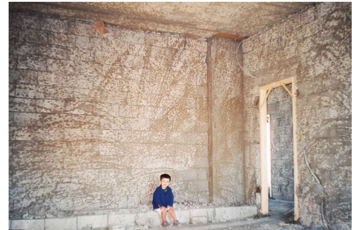
Fig 82. Concrete block visible pre-render, Bedroom 7 on the second floor. Bejjeh, Mount Lebanon. 2001.
