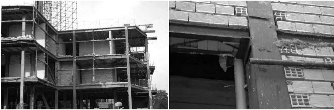
Figure 101. Low building quality in Iran
