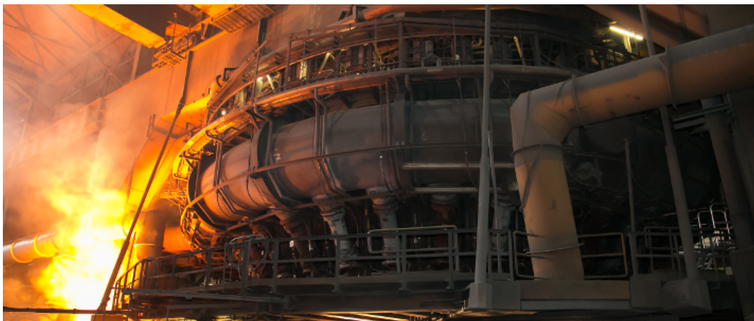
Figure 5.1: Blast furnace A , operated by voestalpine Stahl GmbH in Linz. Lower part of the blast furnace, showing bustle pipe and air distribution manifold [173].
