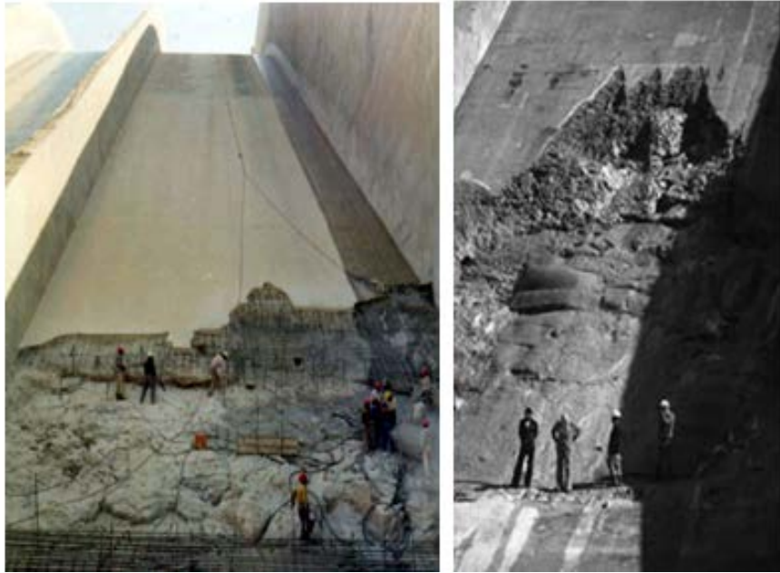
Abb. 21: Kavitationsschäden Karun Dam (Iran) (27, Bureau of Indian Standarts, 2010)
