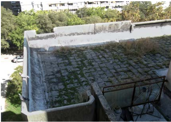
Figure 1 - Natural "green roof" due to poor maintenance
