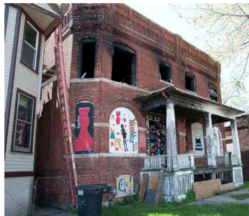
217 Date 24.04.2012, A randomly chosen picture of a gutted building, which could have been nearly anywhere in Detroit
