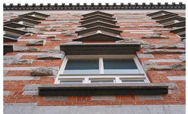
Figure A.319 Slovene National and University Library (1930-1941): close-up view of the façade; present condition ("Jože Plečnik - Narodna in univerzitetna knjižnica")
