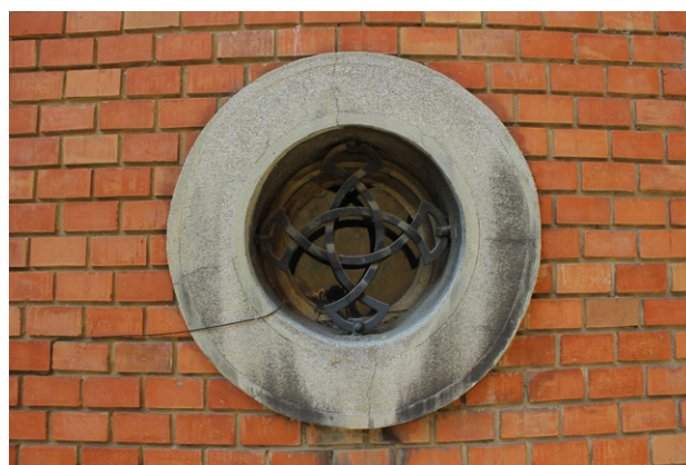
Figure 166 The Parish Church of Saint Anthony of Padua: close-up view of one oculus (2013)
