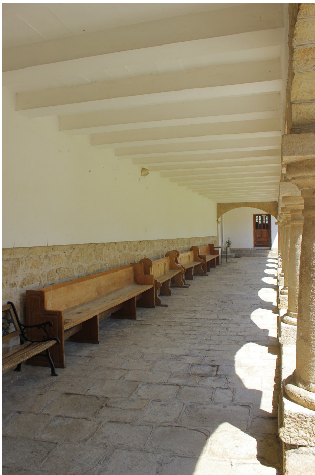
Figure A.98 The Convent of Saint Francis of Assisi, Guča Gora: western cloister hallway (2013)
