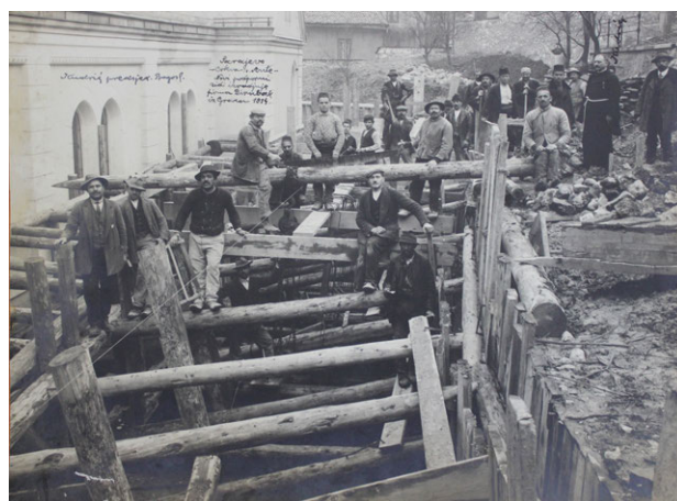
Figure A.23 The convent church of Saint Anthony of Padua, Bistrik: construction works on retaining walls (Archive collection, Petrićevac)
