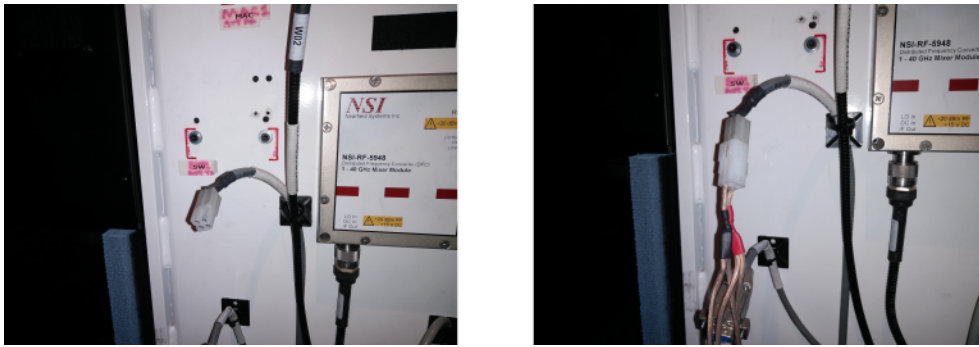
Figure A.3: The end stop sensor connection in unplugged and plugged state.
