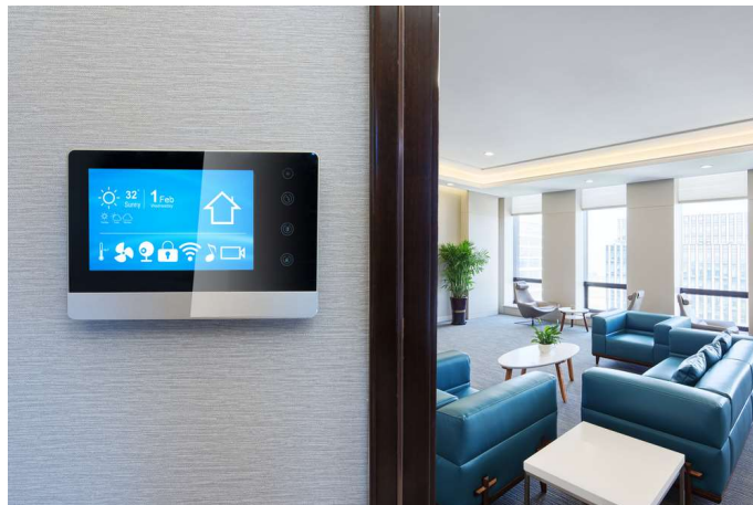
Figure 1: "Smart Home": Control panel in a residential building. 3
