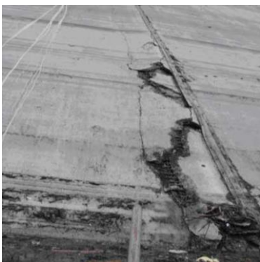
Figure 6 Spalling at joints of Zipingpu CFRD (Chen and Sheng-Shui n.d.)
