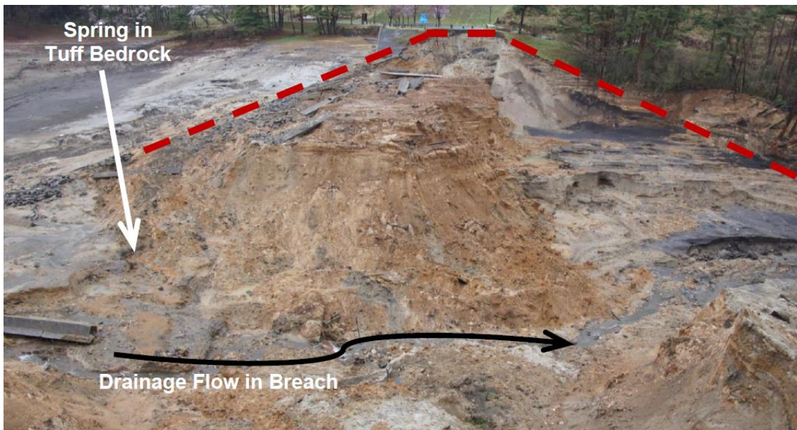
Figure 107 View towards left abutment of breached Fujinuma dam (Harder et al., 2011)
