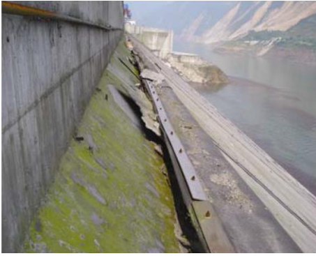
Figure 91 Rupture and spalling of parapet to slab joint (Guan 2009)
