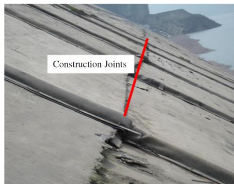
Figure 96 Cold joint failure and slip over of 3 rd phase slab (Chen 2008)
