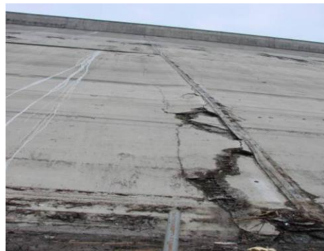
Figure 94 Massive spalling off of concrete edges at vertical slab joints (Chen 2008)
