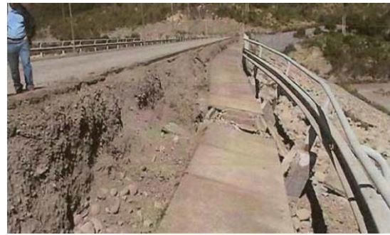
Figure 5 Slides close to the crest of Colbun dam (Nogueira 2010)
