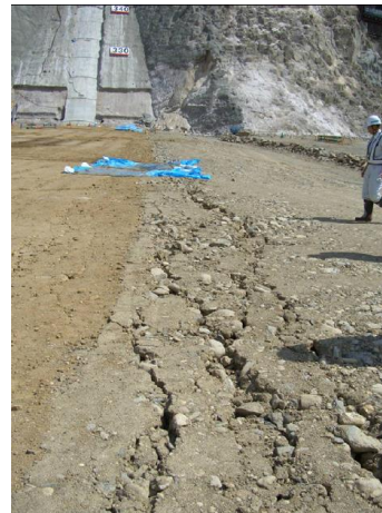
Figure 43 Close up of cracks in Isawa dam (Shimamoto et.al. 2008)
