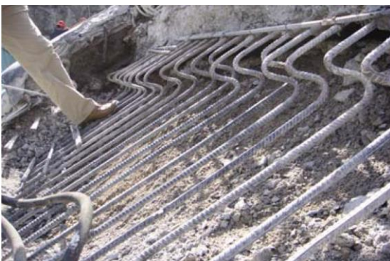
Figure 95 Repair works at cold joint slip over of 3 rd phase slab after concrete removal (Guan 2009)
