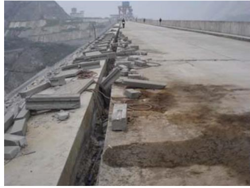
Figure 92 Dislocation of pavement at the crest's edge (Guan 2009)
