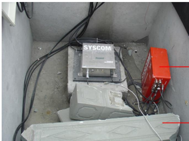
Figure 133 Crest accelerograph hit by destroyed unreinforced concrete guard elements (Zou 2012)
