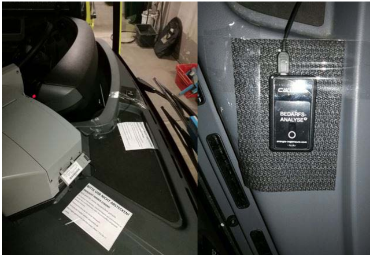
Figure 21: Installation of logger in the Mercedes Citaro on line 501
