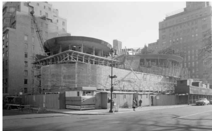
Fig. 2. 2 Architecture Guggenheim Museum, New York City, F. L. Wright: Construction process (Gottscho-Schleisner, 12 November 1957)
