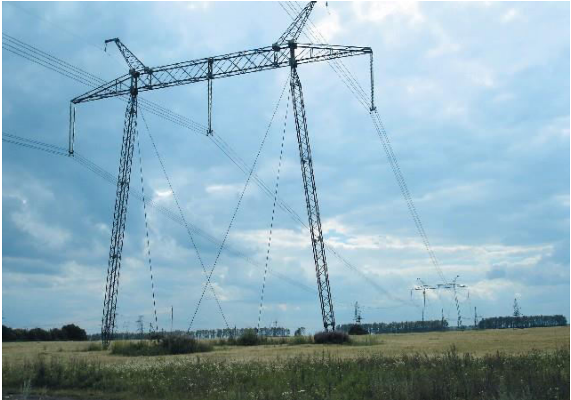
Figure 2. High-voltage transmission lines 750 kV
