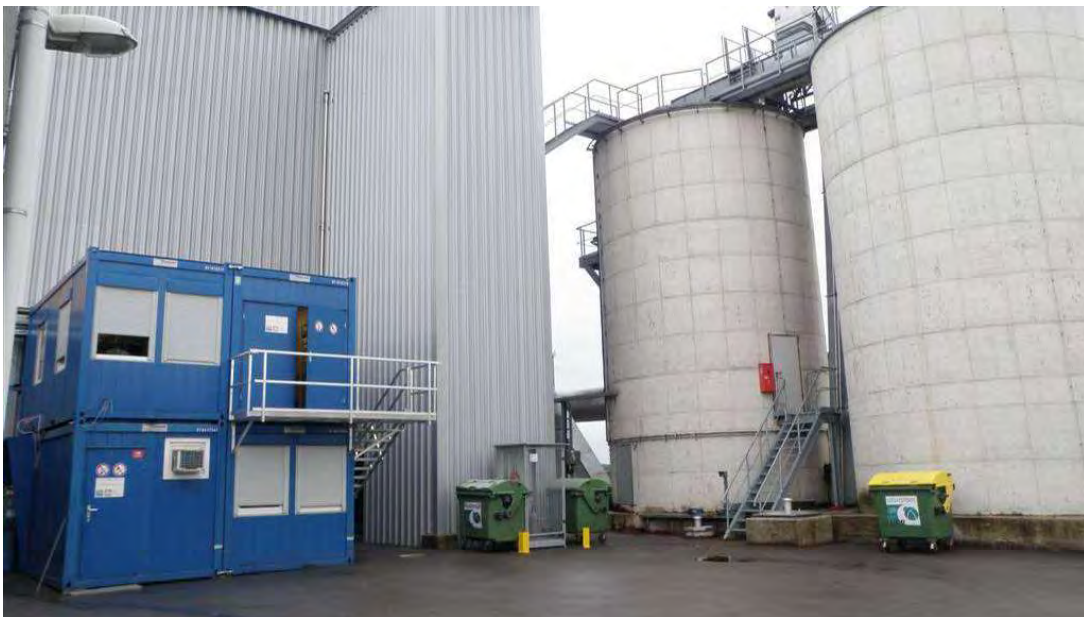
Figure 4.6: Picture of research containers next to the DFB biomass steam gasification power plant Oberwart in 2014; in the container on bottom a series of analytical devices were placed; in the container on top a series of pilot plants for wood gas processing were realized.
