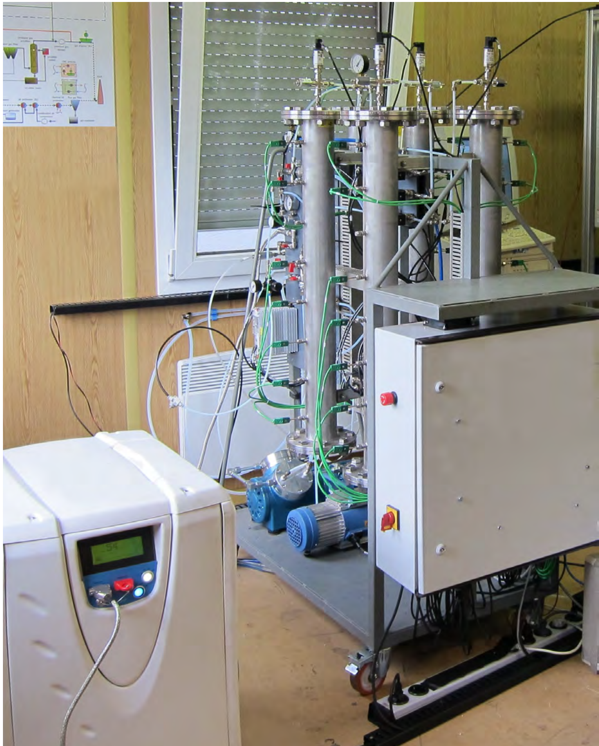
Figure 3: S3 – Left: PEM fuel cell for the demonstration of the quality of the generated BioH 2 ; Right: PSA unit employed for H 2 separation of the preconditioned wood gas.
