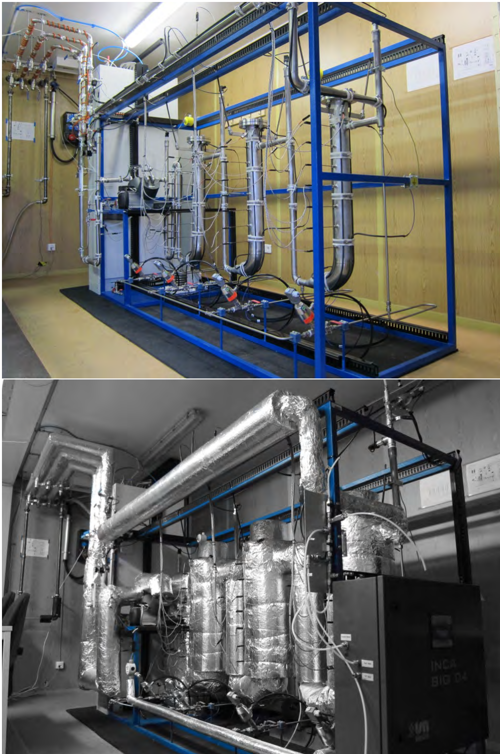
Figure 5.6: Pictures of the realized "Pilot plant for catalytic wood gas processing" (WGS unit); top: picture prior to heat insulation 2012; bottom: picture of the final setup in 2013, including heat insulation, sampling for gas analysis, etc.
