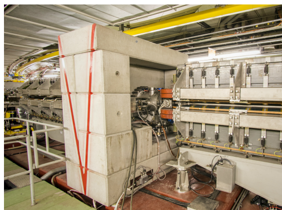
(c) Photo of the installation in the tunnel.
