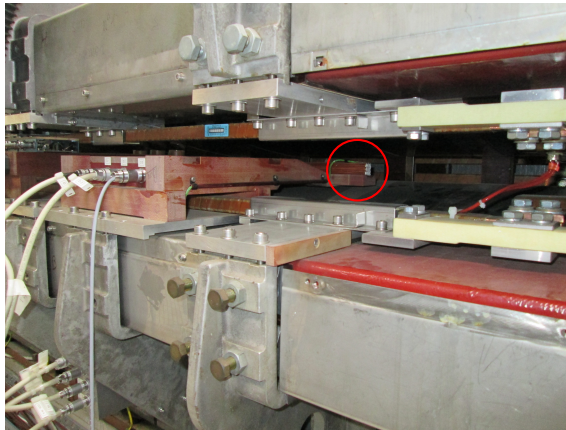
(a) Installation of the coils inside the focusing half-unit of MU101. Their location is indicated by the red circle.
