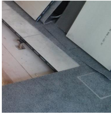
Figure 7. The picture shows an opening of a raised floor system, Palais von Foerster
