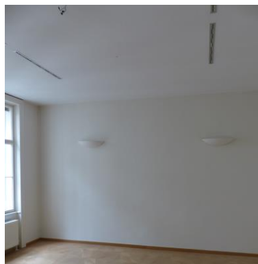
a.) Gypsum cardboard suspended ceiling
