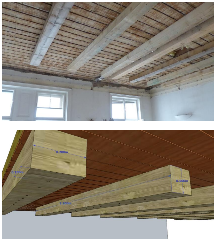
Figure 23. Third refurbished construction (e), wooden beam “stiffeners” bolted on the original wooden beam structure with 200x6 mm bolts every 150 mm.
