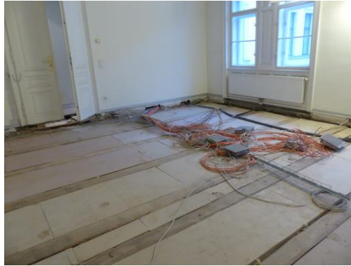
Figure 17. Level 4, floor after removing the layers on top of the wooden beam construction
