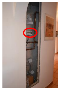
Figure 17. EWT Scylar Int 8 mounted at the storage tank.
