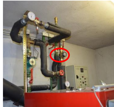
Figure 15. EWT Ray heat meter installed at pellet furnace.
