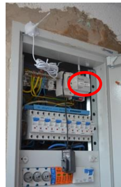
Figure 21. Thermokon SR-MI-HS installed in the fuse box of NAT.
