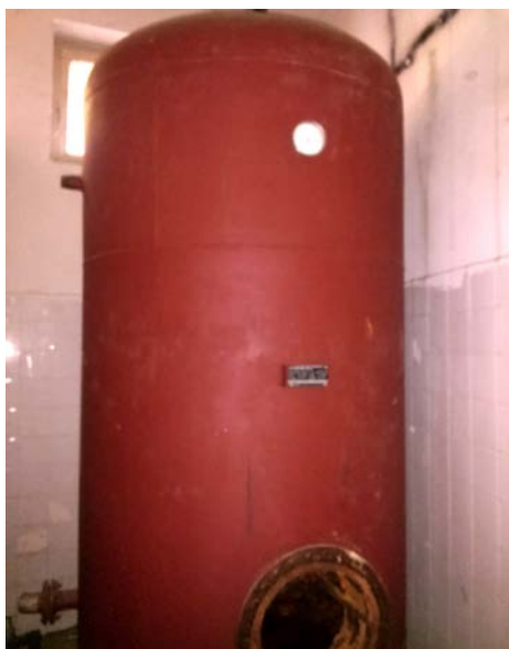
Abb. 85 Hydrophon in Raum 14
