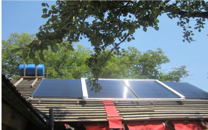
Figure 8: Installed vacuum tube collectors in Böheimkirchen prototype house – GrAT
