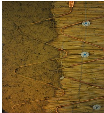
Figure 9: Wall heating system which has been installed in the prototype house- Böheimkirchen
