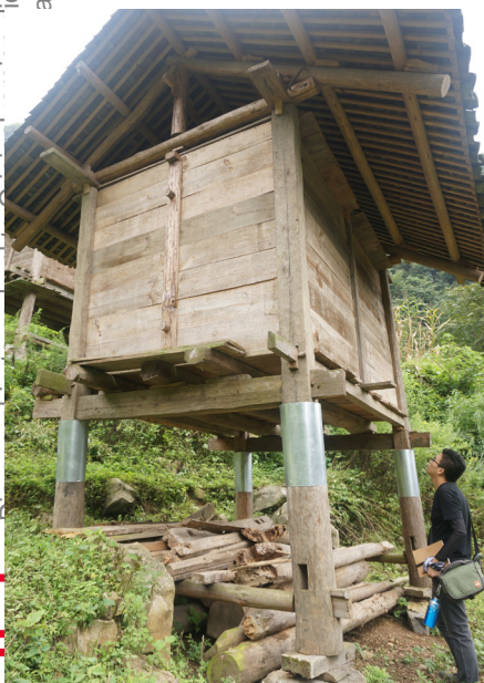
Fig.4. 34 Thin aluminium sheets were wrapped on the upper parts of posts of the granary.
