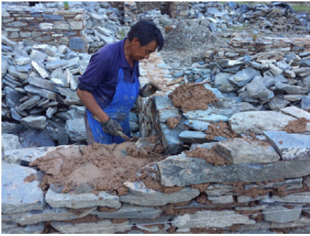
Fig.6. 7 A Tibetan mason was working on a building site, Cong'en, Sha'er Zhong, Sichuan.
