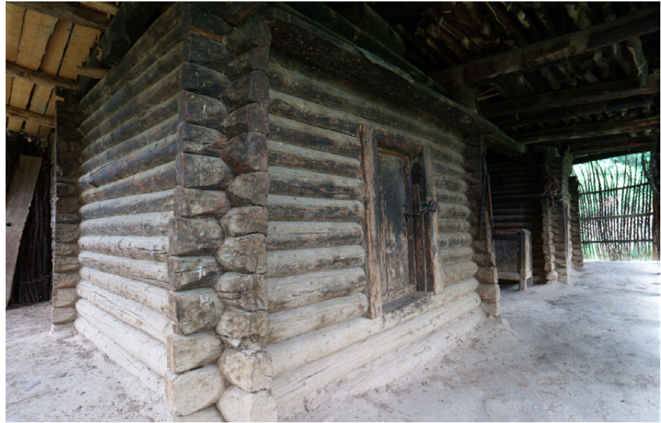
Fig.6. 34 Two log granaries on the 5 th floor of Ke Sha house. (source: Klaus WERGER)
