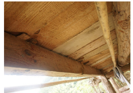
Fig.4. 31 Thin wooden blocks were inserted between the floor and lower beams beneath as a remedy measure.
