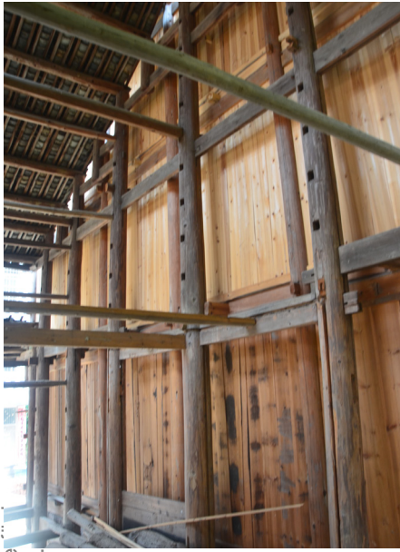
Fig. 4.83 A damaged framework of a granary.
