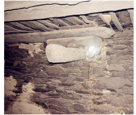
Fig.6. 42 The inner ends of the cantilevered beams are mainly pressed by wooden blocks or short beams beneath the ceiling.
