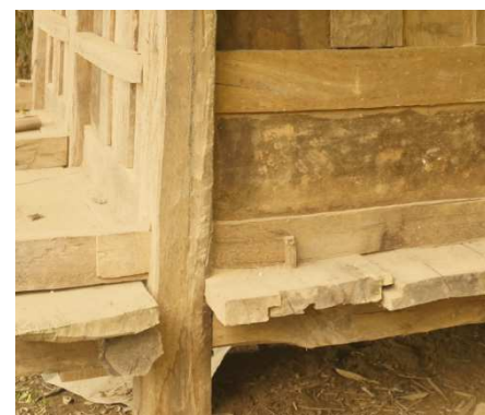
Fig.5. 44 Wooden nails were added vertically along the edges of the beams for impeding their outward pressure
