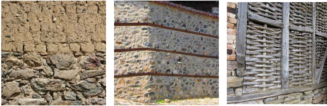
Fig. 63: Textures, extracted from Bulgarian villages: a) adobe bricks on stone foundation, b) wall with rock stones on a clay composition with levelling timbers and c) wattle fence elements.
