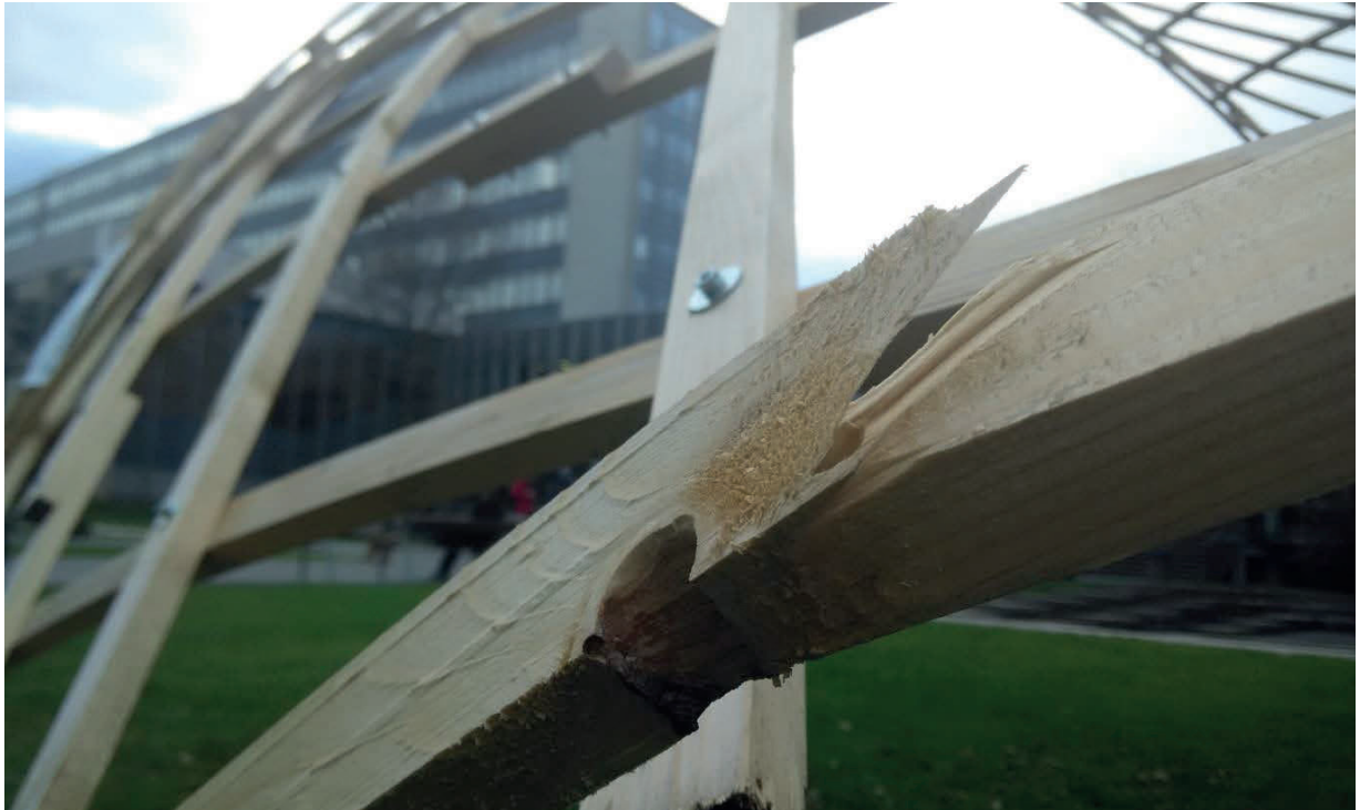
Fig. 3.4 Example of material failure caused by fast erection (in place of material imperfection)
